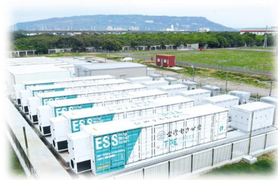
儲能系統 (Energy Storage System, ESS)
