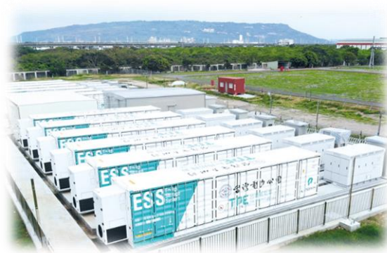
儲能系統 (ESS, Energy Storage System)
